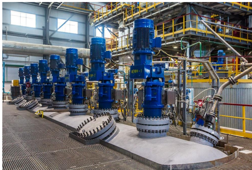
Autoclave at Amursk POX plant
